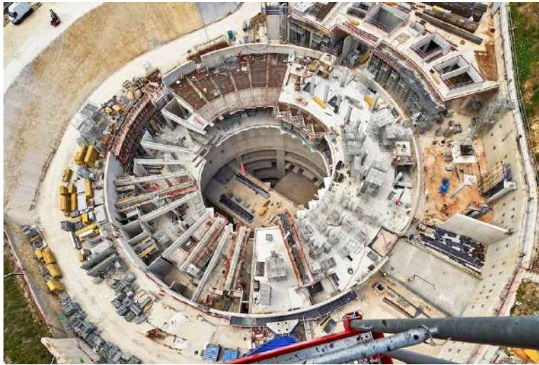
The Villejuif Institut Gustave-Roussy station is located in the Hautes-Bruyères park to the South of ... [+] © MICHEL DENANCÉ, DOMINIQUE PERRAULT ARCHITECTE, ADAGP 2021
